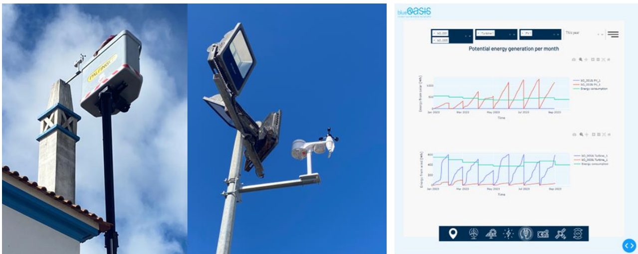
Figure 1: Left - Sensors at Ericeira Business Factory; Right - Snapshot of the existing dashboard.
